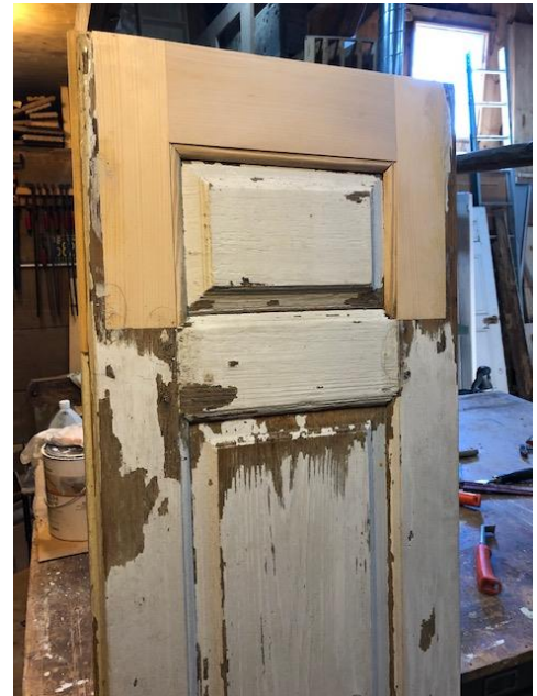
Substantial efforts were made to preserve as much original fabric as possible in repairing the 1783 shutters. --¶
