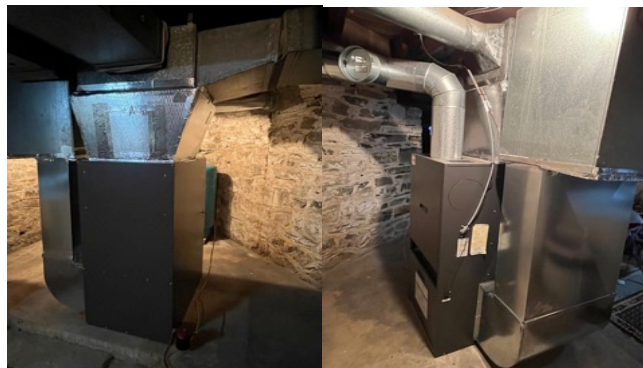
New furnace installed in November 2025.
